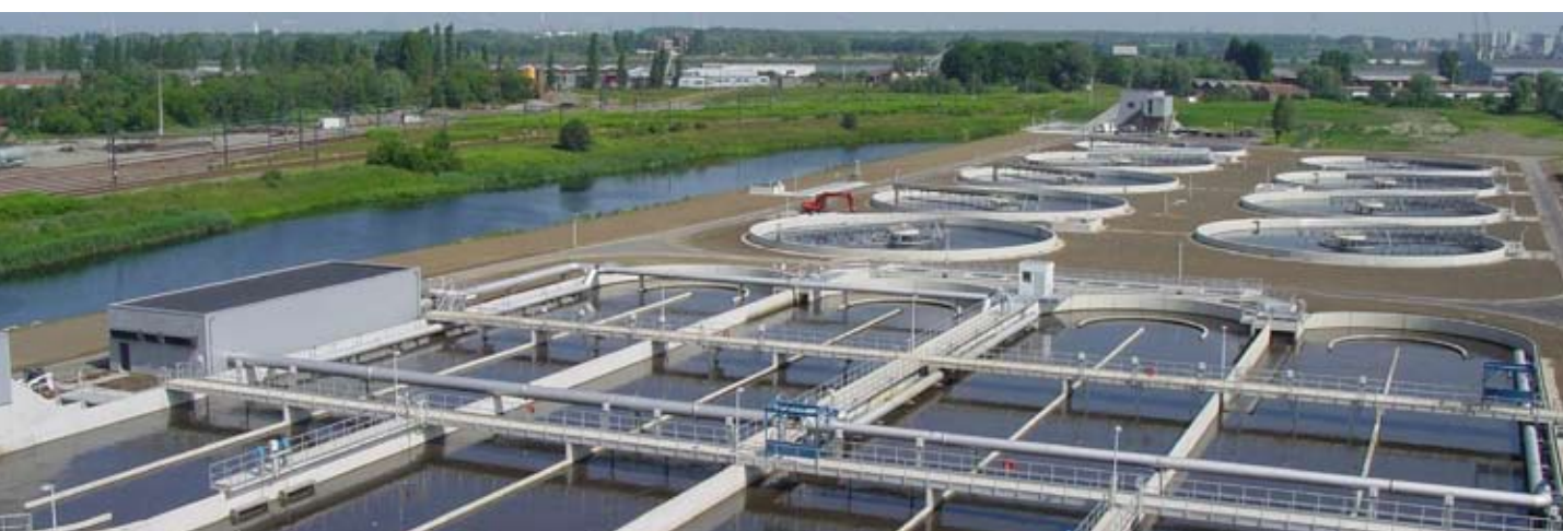
Wastewater Treatment - Belgium
